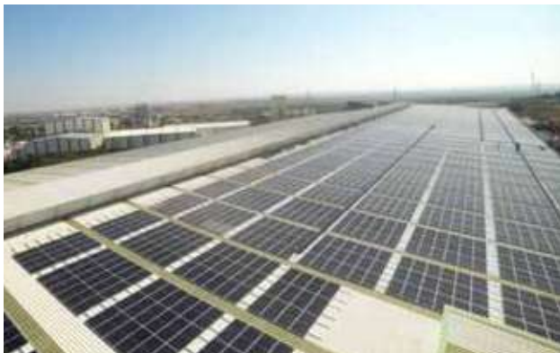
Solar Power Plant commissioned successfully at Nooriabad Factory, Sindh
