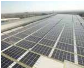
Commissioned 2MV On-Grid Solar Power Plant at its manufacturing facility at Nooriabad
